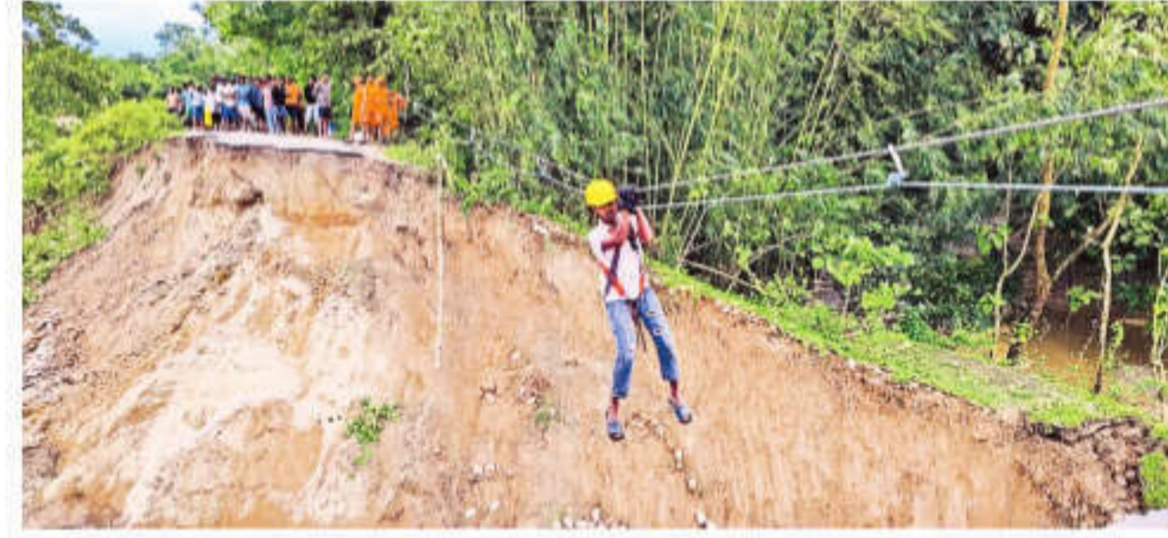
Rescue operations underway after a bridge collapsed in a landslide-hit area following heavy rainfall in Darjeeling, on Sunday. NDRF via PTI
